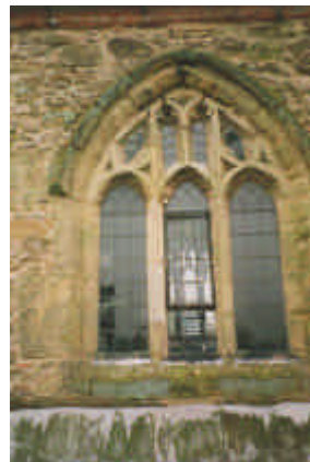
13. These photographs show the extent of the damage to the tracery of the clerestory windows. During the repair of the trusses and whilst the scaffolding was in place
