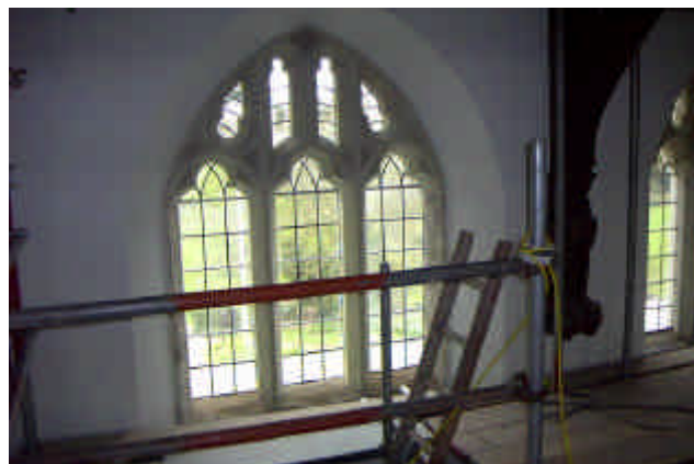
14. It was decided that during the repair of the trusses and whilst the scaffolding was in place (internally) that repairs should be made to the tracery
